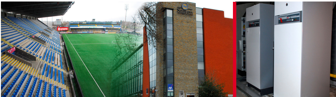
HeatMaster® TC cascade-opstelling in complex Hotel Stayen (Sint-Truiden)
